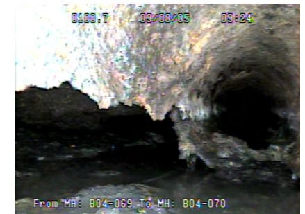
Hole Due to Corrosion
