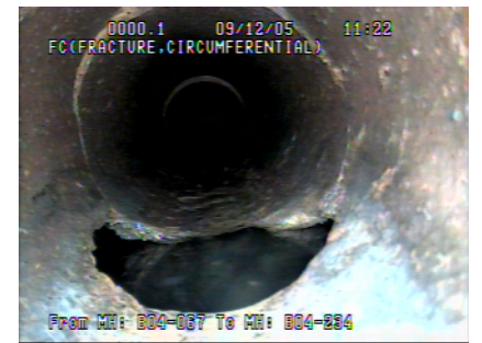
Hole in Pipe
